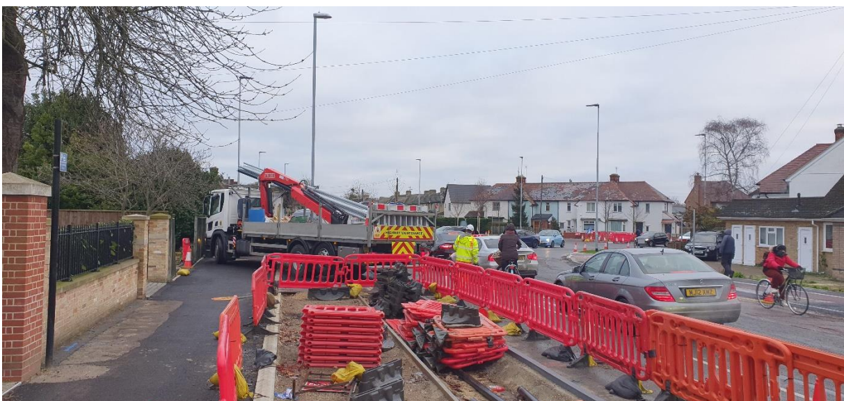
Photo: View of the works at the south-west approach to the Elizabeth Way / Highworth Avenue roundabout
