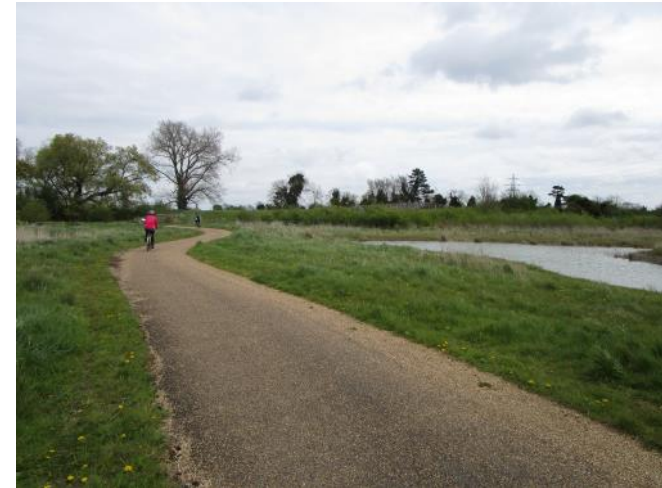
Tar spray and chippings were added to a sealed blacktop surface on this path near Lode.
